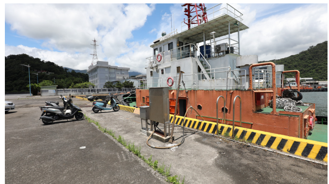
Vessel Use of Shore Power
