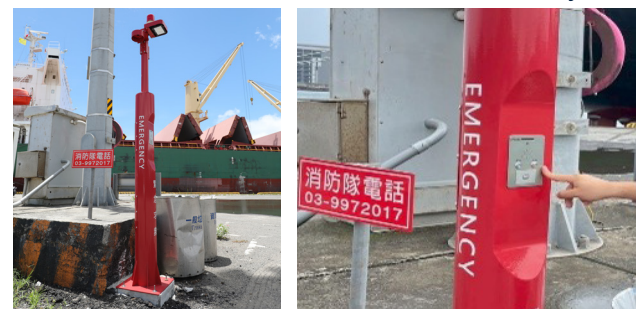
Functionality test of the smart emergency call tower
