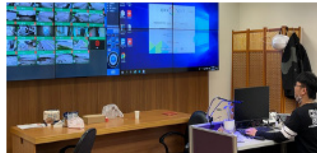
The Port of Su-Ao monitors port conditions in real time through CCTV surveillance systems
